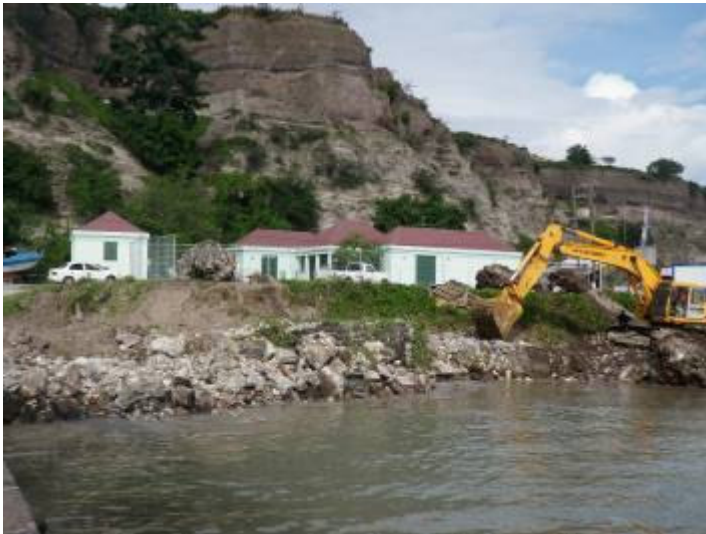
Work begins on the dingy and dive dock in Lower Town. Ruins have been partially recovered and stored for integration in a later phase of the project.
